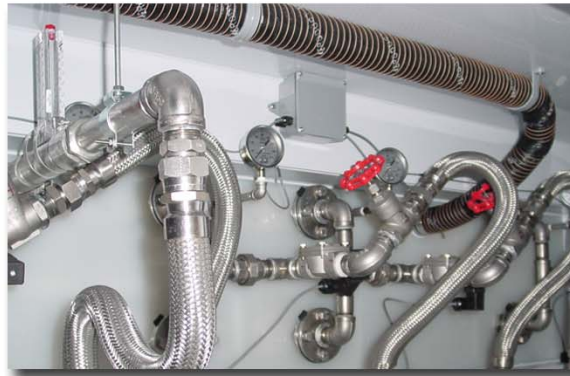
Stainless Steel Plumbing and Pressure Gauges
